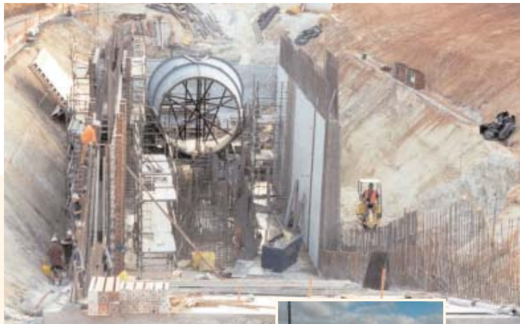
Above: Pacific Hydro's power generation plant at The Drop, near Berrigan, pictured here under construction.
